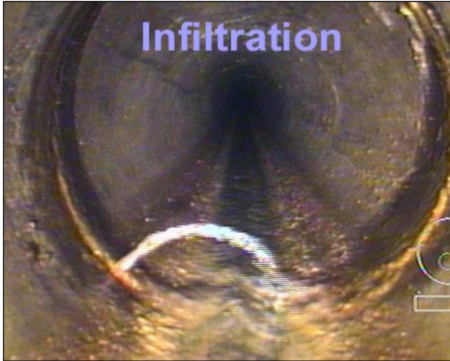
Figure 9.95 Example of infiltration into a sanitary sewer network (courtesy City of Surrey, Canada)
