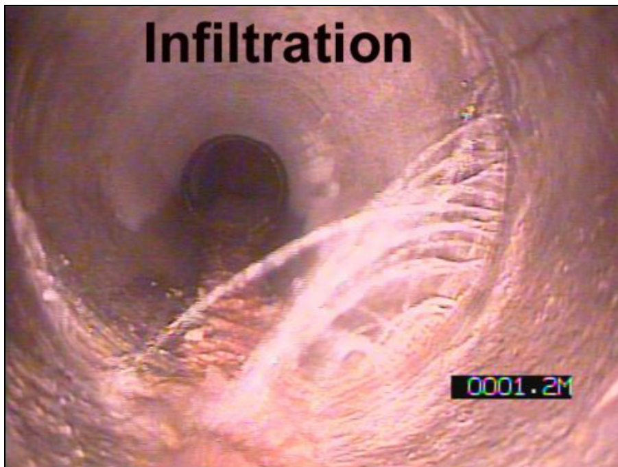
Figure 9.96 Example of infiltration into a sanitary sewer network (courtesy City of Surrey, Canada)
