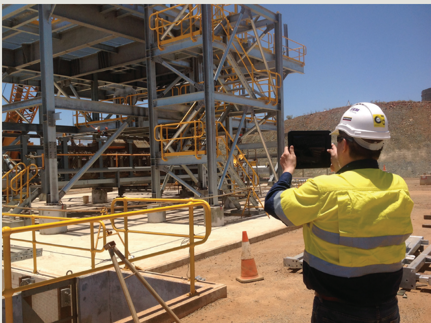
Use of a tablet computer onsite allows the project team to view the project's 3D model, as well as access work packs (library of 2D, 3D and specification information), construction check sheets, and defects and issues reporting.
